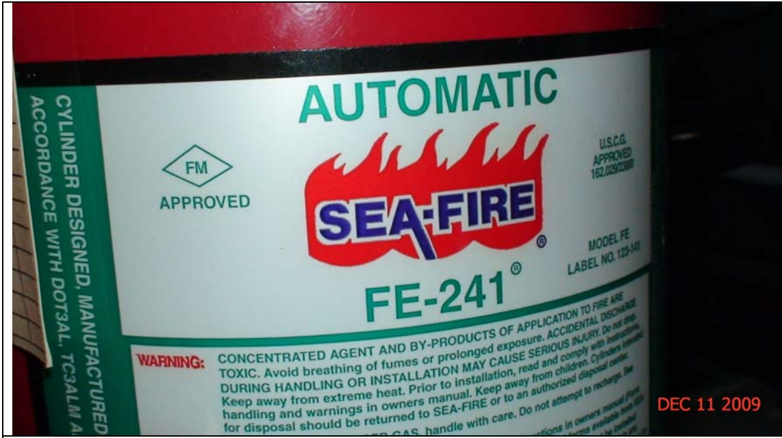
Signage for fixed fire extinguishing system.
