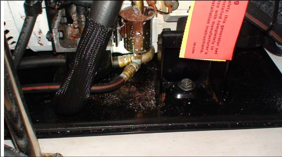
Slight corrosion in ONAN generator housing. Preventative maintenance needed.
