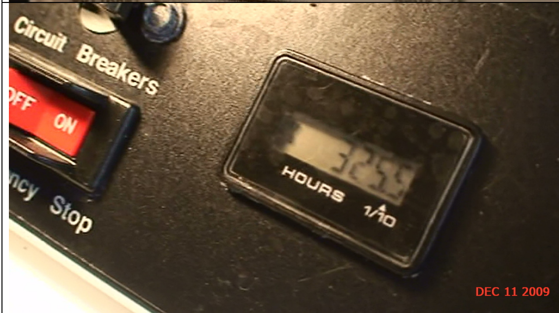
ONAN diesel generator engine placard and LCD hour meter showing 325.5 hours.
