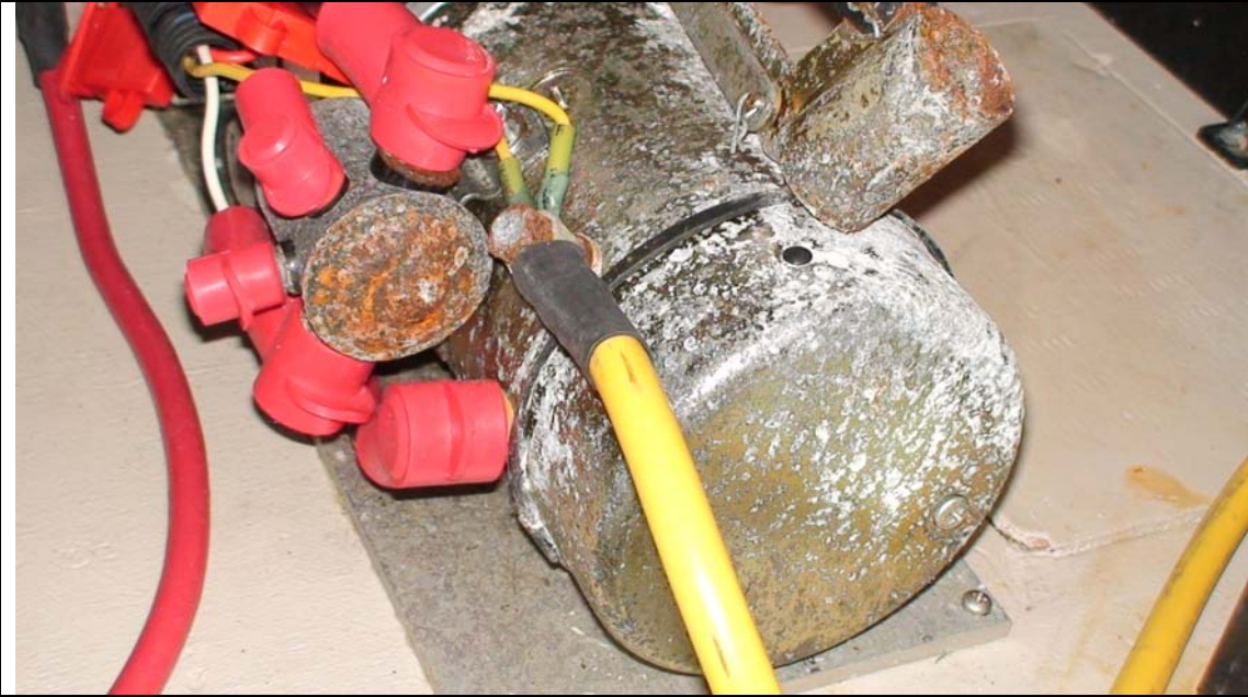
Surface corrosion on hydraulic dinghy lift. Preventative maintenance needed.
