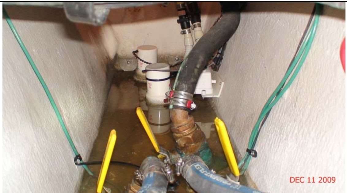
Aft bilge showing readily accessible seacocks and aft bilge pumps.
